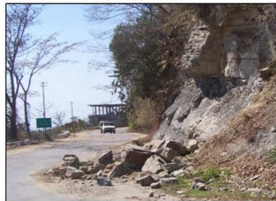
Plate 2 : Road cutting without considering slope stability causes rock fall near Kolasib town, Kolasib district.
